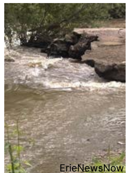
Centerville Dam Post Blowout
